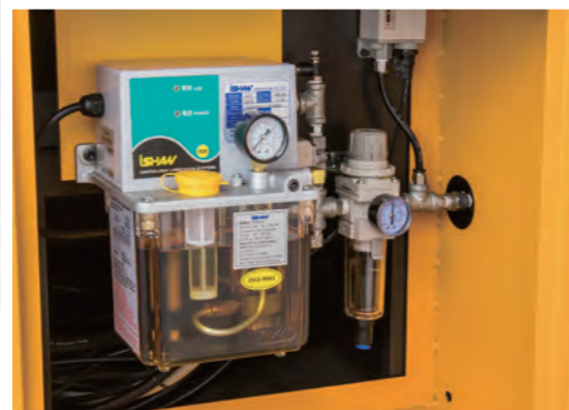
Automatic lubrication unit.
